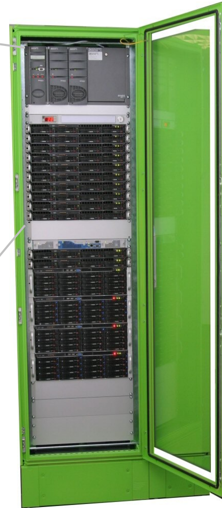
A-Server “Datacenter in a rack”
